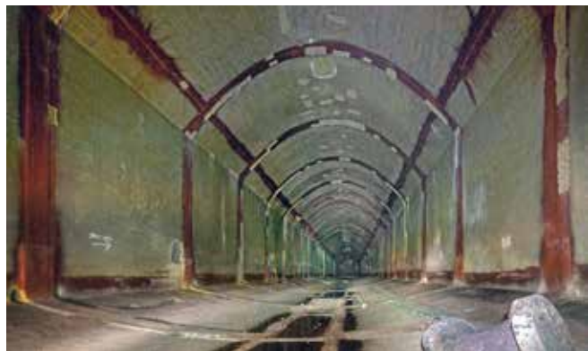
Inside tank no. 4 – part of the dismantled fuel pipe rests on the floor tanks could each hold 25 million litres of furnace fuel oil. Construction here was completed much quicker, and
